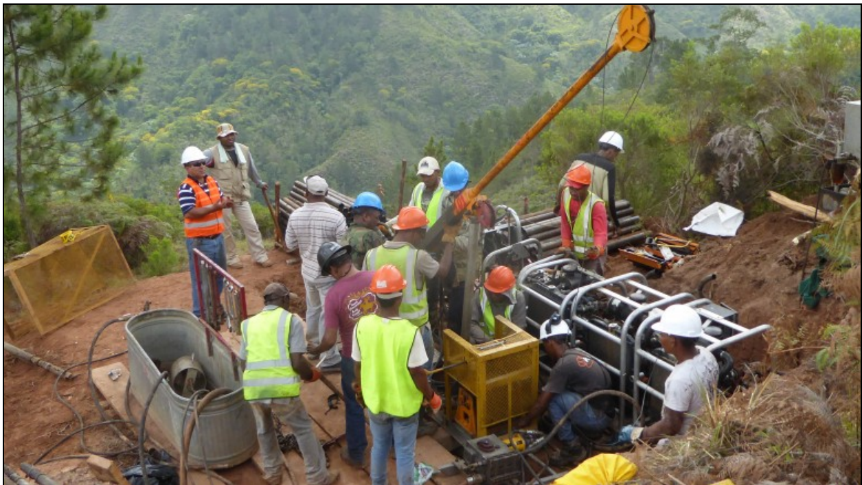
Drill crews work at the Ginger Ridge target on the Juan de Herrera gold project in the Dominican Republic. Credit: Precipitate Gold.
